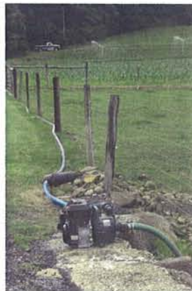
IRRIGATION AND SOLUTION TRANSFER
